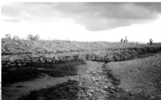
Spurs constructed along the rivulets in Ilam district have helped prevent crop damage during the monsoon
